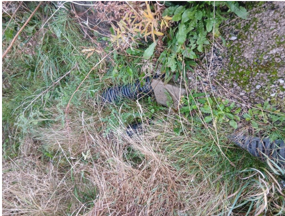
Photo 7 — Drainage running through the ditch.
