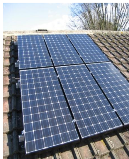
Figure 8 - Photovoltaic array on a pitched roof
