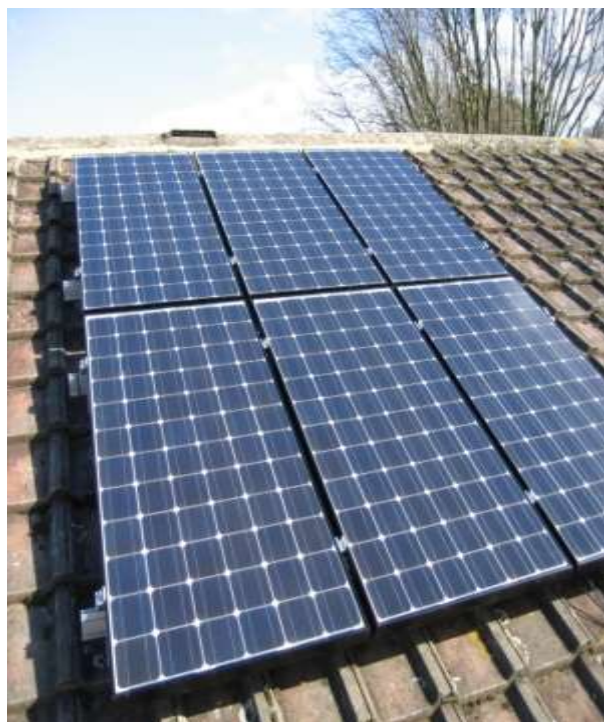
Figure 10 - Photovoltaic array on a pitched roof
