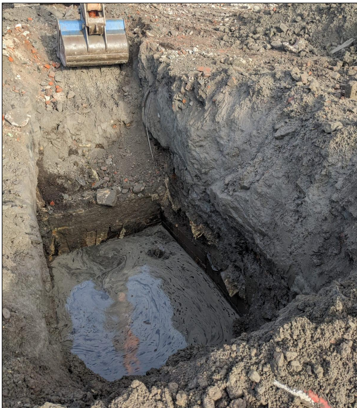
Plate 9: Flooding during excavation, looking north
