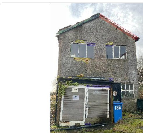
Photo 1: Annotated image of the northern face of the building. Purple – gaps, Yellow – Exposed brick with missing mortar and Red – missing fascia.
