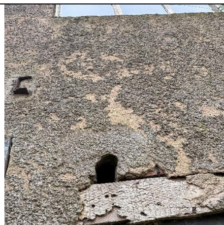
Photo 14: Gap above door. Northern face
