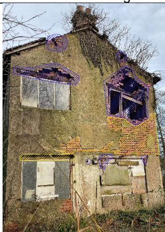
Photo 3: Annotated image of the southern face of the building. Purple – gaps and Yellow – Exposed brick with missing mortar.
