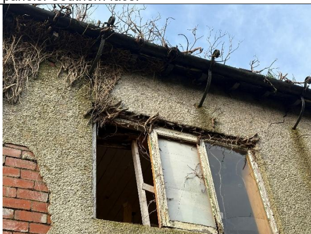
Photo 11: Missing windowpane. Eastern face.
