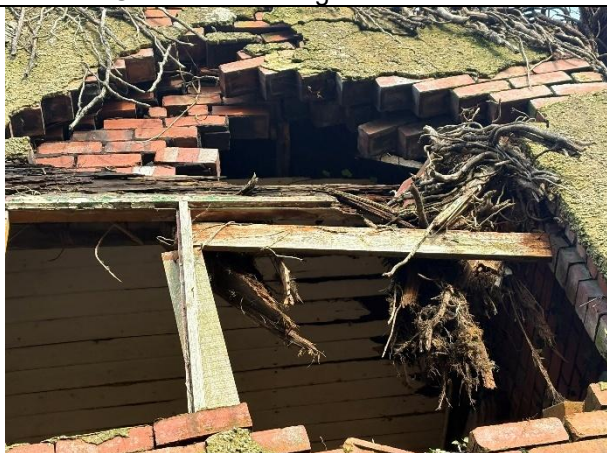
Photo 9: Exposed cavity into house and gaps in roof panels. Southern face.
