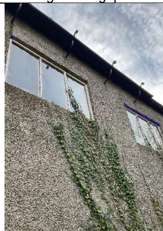
Photo 4: Annotated image of the western face of the building. Purple – gaps.
