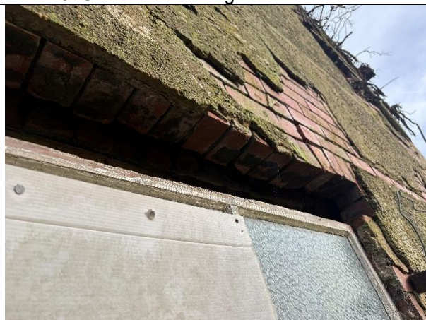
Photo 10: Gap above windows. Southern face.
