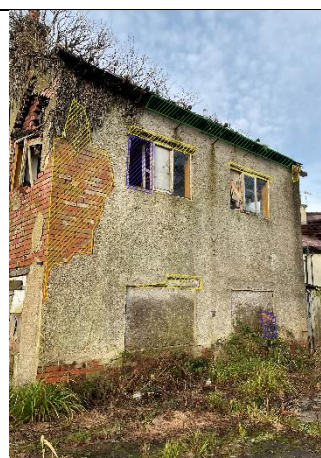
Photo 2: Annotated image of the eastern face of the building. Purple – gaps, Yellow – Exposed brick with missing mortar and green is gaps in soffit.
