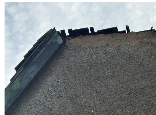
Photo 13: Missing fascia. Northern face.
