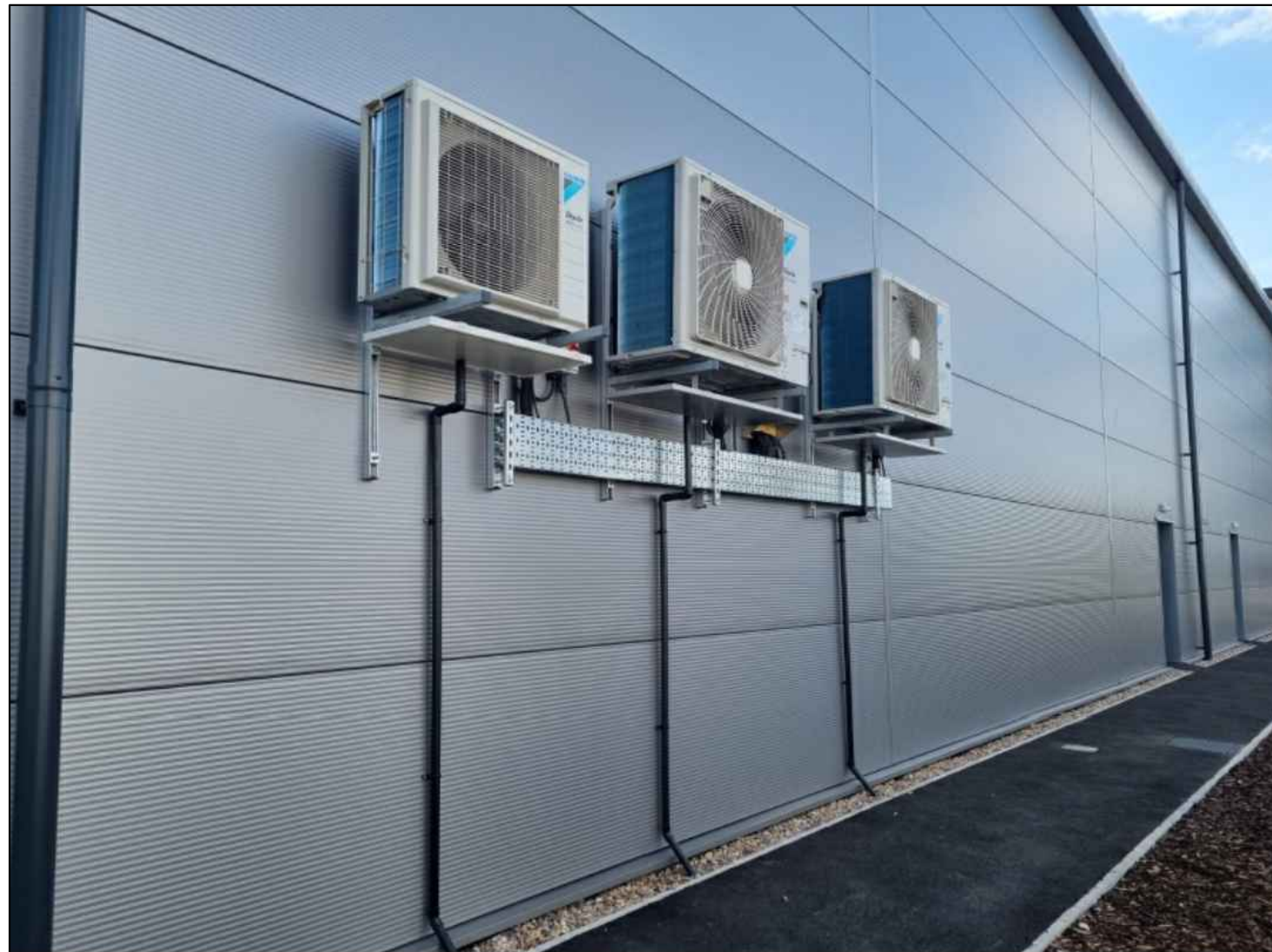
PHOTO OF TYPICAL ASHP CONDENSER UNITS MOUNTED AT HIGH LEVEL NOT TO SCALE
