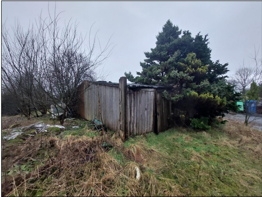
View of Dilapidated Outbuilding (Facing North East)
