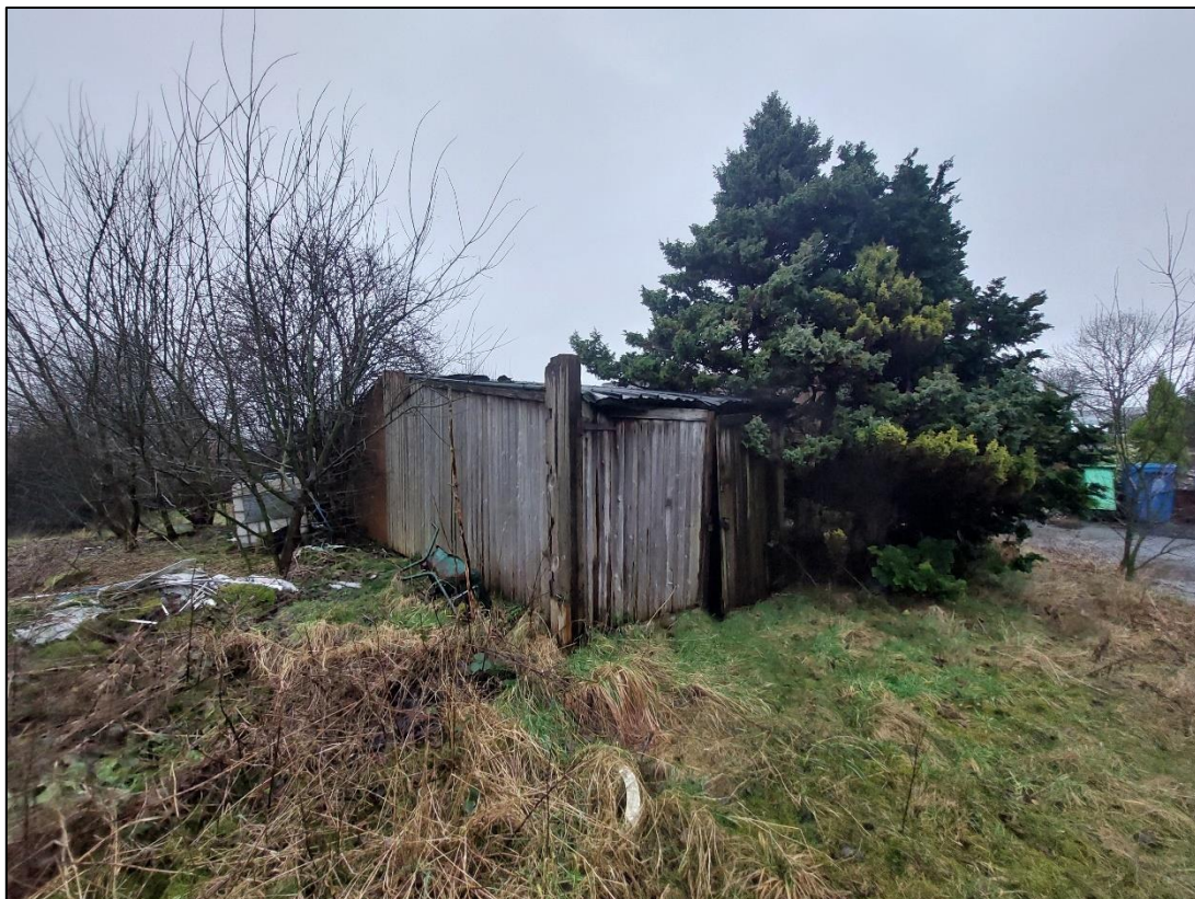
View of Dilapidated Outbuilding (Facing North East)
