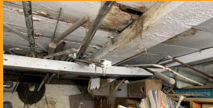
Damage in main barn
