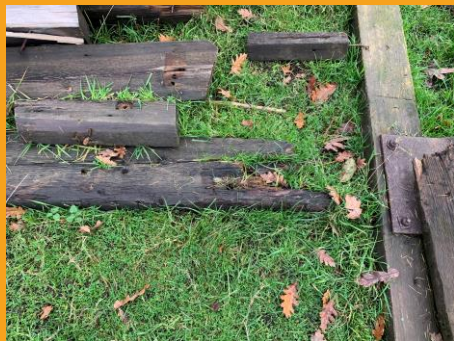
Damage to roof timbers
