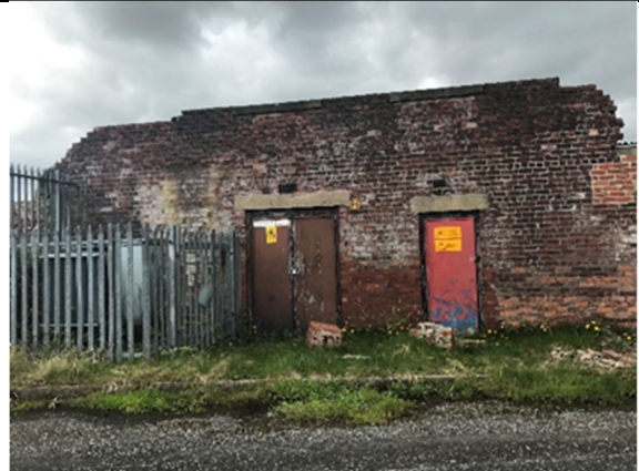
Photograph 11: Live electricity substation in the north-east of site.
