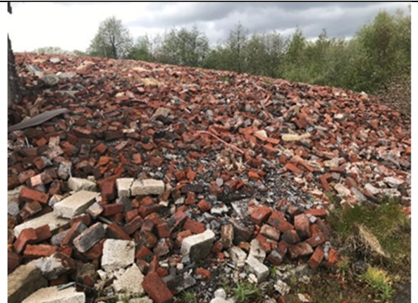
Photograph 10: Ash and demolition rubble adjacent to access road into the site behind containers and electricity substation, north-east of site.
