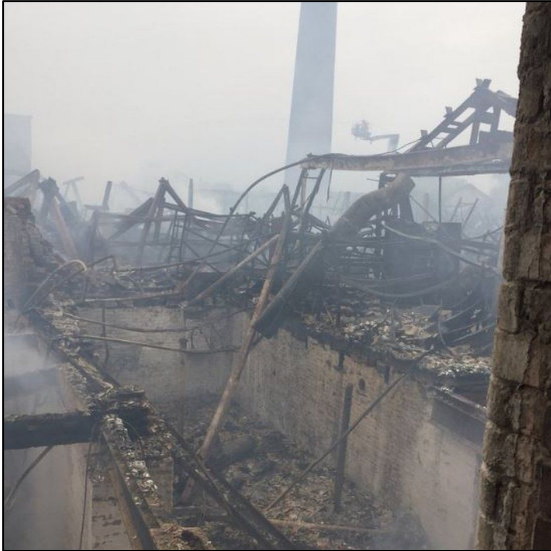
Plate 2-4: Mill building and chimney following fire 5 .
