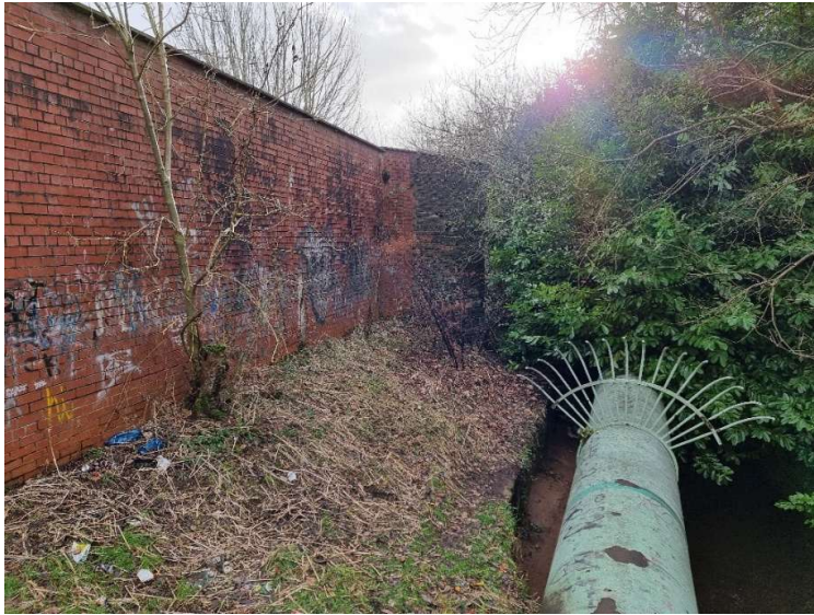
Photograph 3 – South West corner of application site with Sudden Brook running approximately 1.8m lower than the base of the masonry wall that encloses the yard serving the application site.
