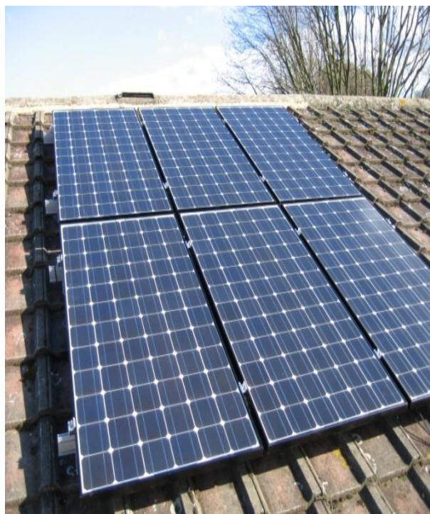
Figure 9 - Photovoltaic array on a pitched roof
