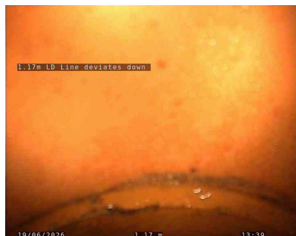
4, 00:00:22, 1.17 m Line deviates down
