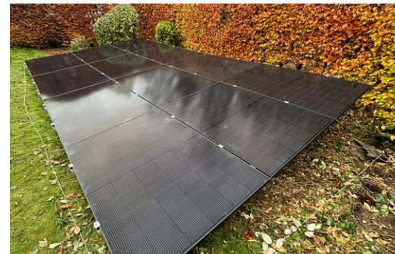
screened ground mounted solar
