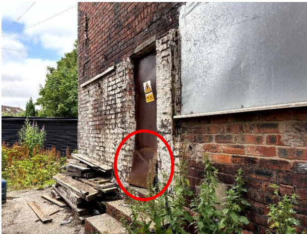
Gable wall and evidence of damage to doorway sheeting where unauthorised entry had occurred
