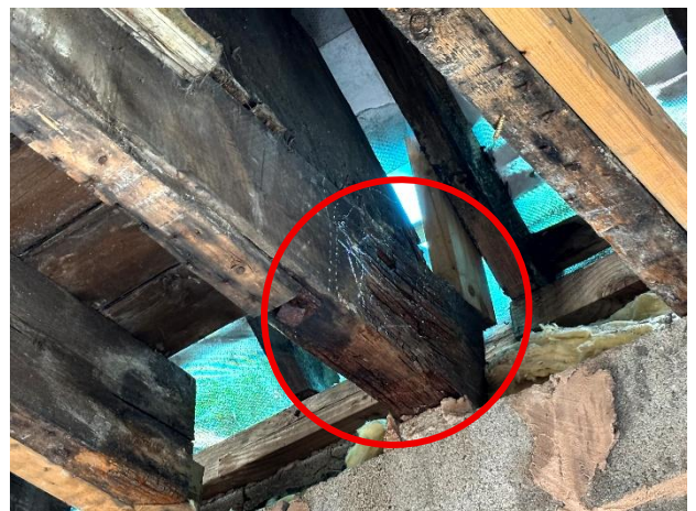
Water ingress affecting rear truss bearing
