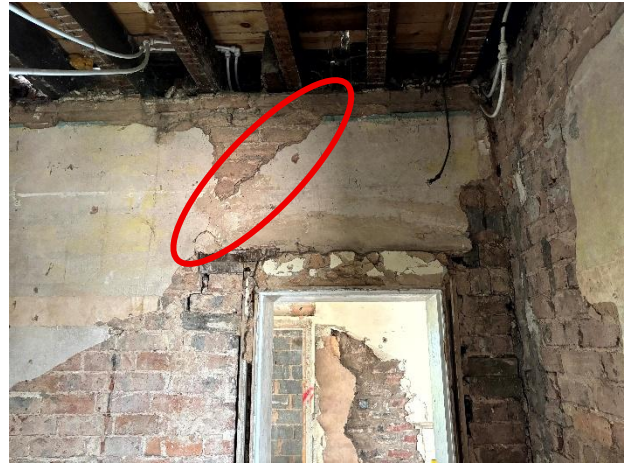
Cracking above doorway into stairwell from front lefthand room
