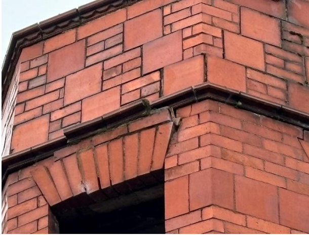
Rotated brick arch noted in 2024
