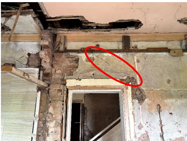
Cracking above doorway into stairwell from rear lefthand room
