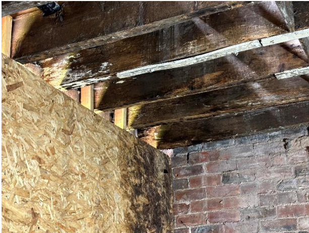
Deterioration of timber due to water ingress in front lefthand corner
