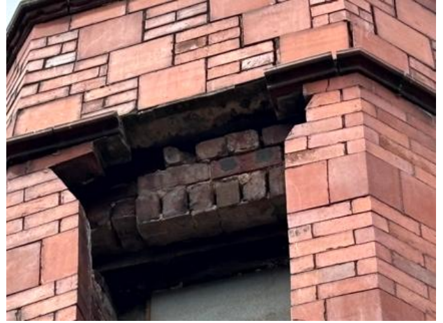
Brick arch missing in 2026
