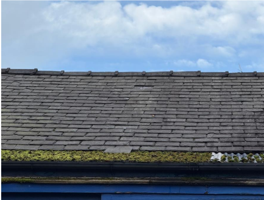
Lifted and missing tiles
