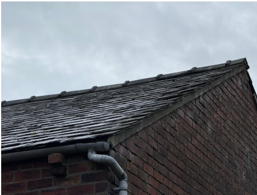
Gaps in ridge tiles
