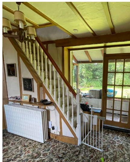
Fig.20 - Existing steep stairs
