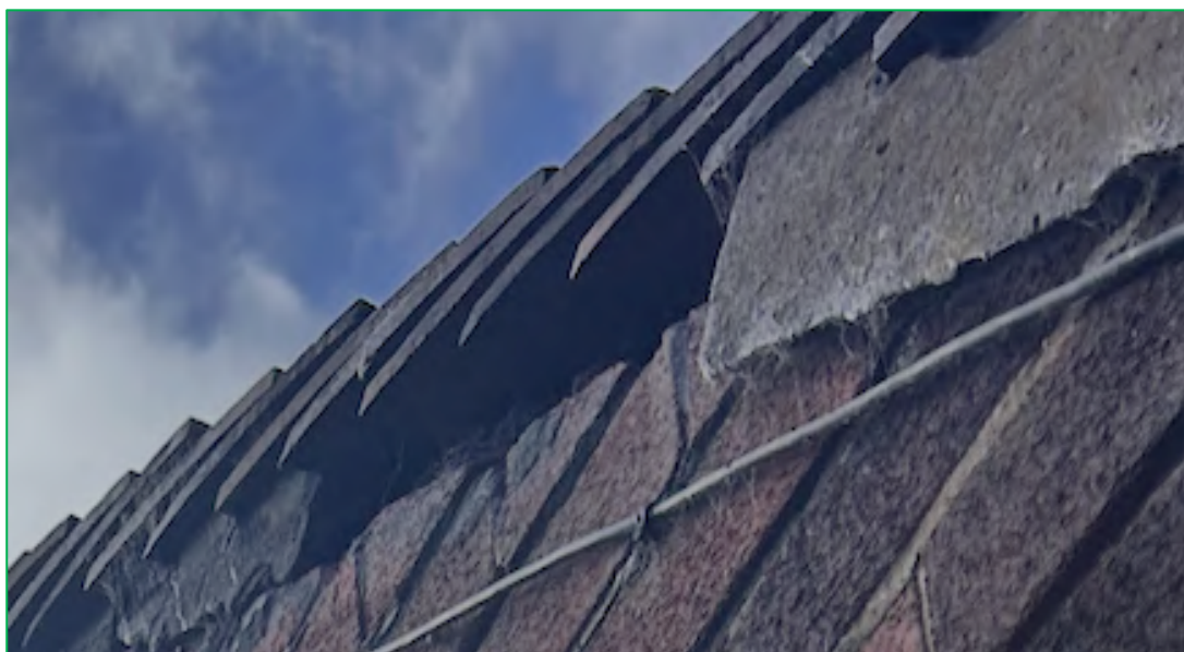
Large gap in the gable on the east elevation
