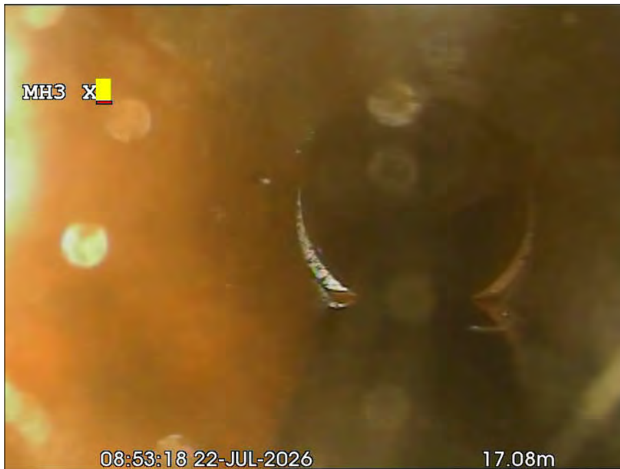
Photo: 11_7a, 00:00:00 17.5m, Joint displaced. Medium
