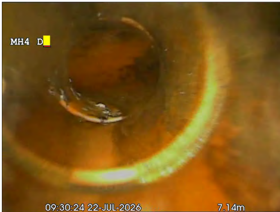
Photo: 18_7a, 00:00:00 7.2m, Joint displaced. Medium
