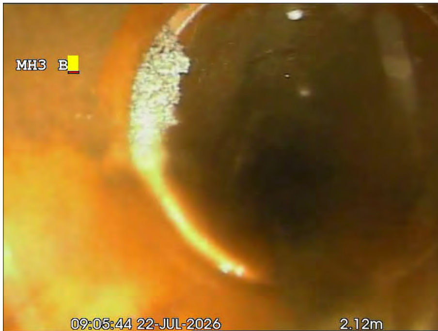
Photo: 7_5a, 00:00:00 2.2m, Joint displaced. Medium
