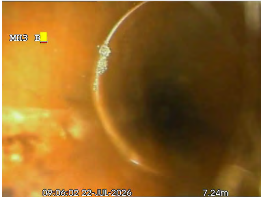
Photo: 60_10a, 00:00:00 7.3m, Joint displaced. Medium
