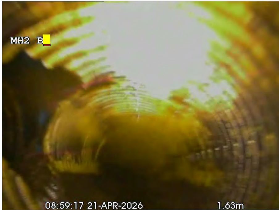
Photo: 279_4a, 00:00:00 1.6m, Connection, at 09 o'clock, dia 80 mm
