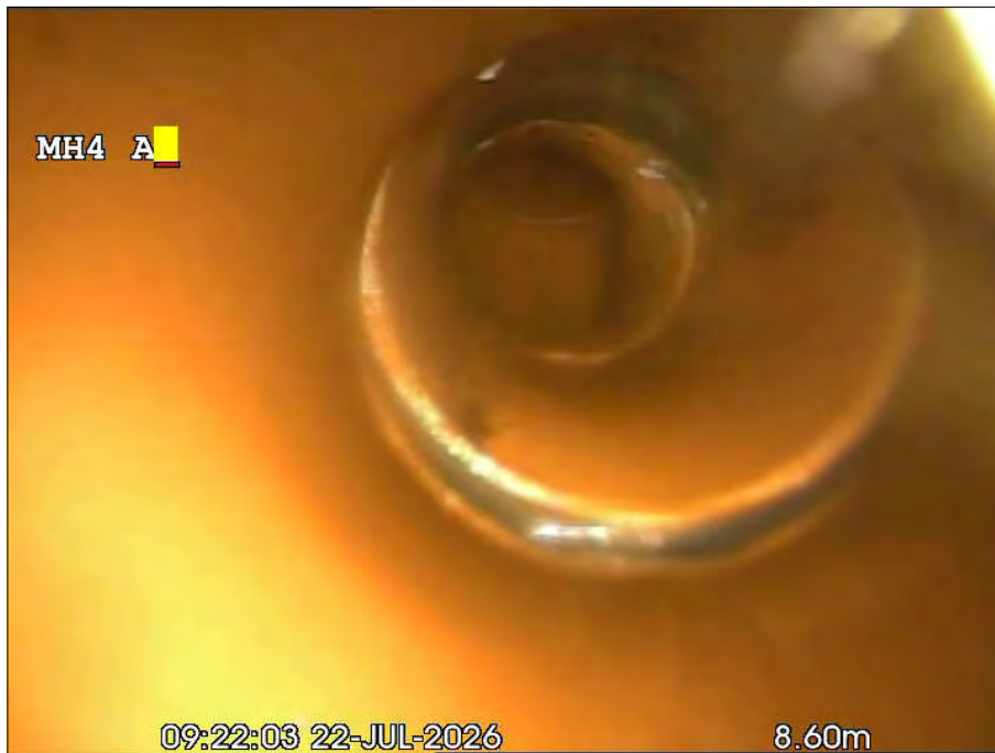
Photo: 12_5a, 00:00:00 8.4m, Joint displaced. Large
