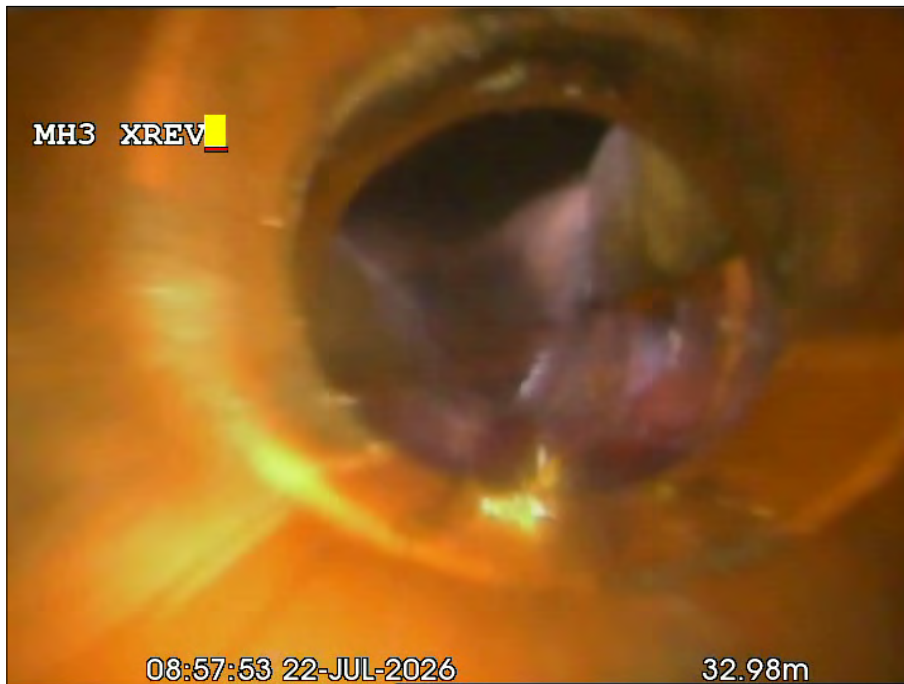
Photo: 11_14a, 00:00:00 34.1m, Joint displaced. Medium
