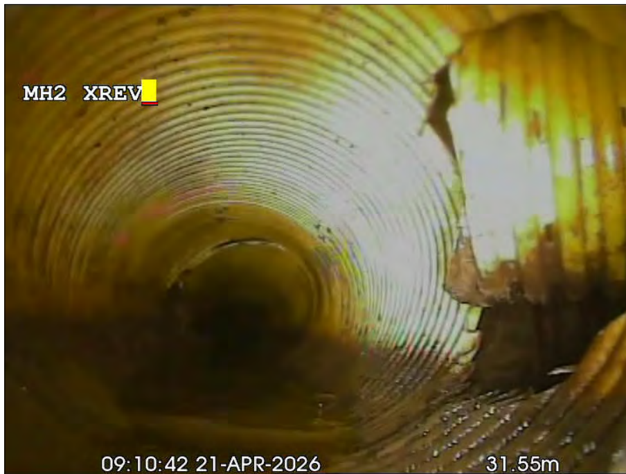
Photo: 34_14a, 00:00:00 31.9m, Connection, at 03 o'clock, dia 80 mm
