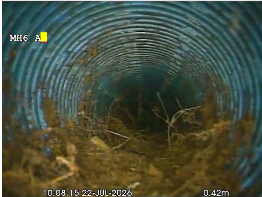
Photo: 256_4a, 00:00:00 0.5m, Debris silt, 5 % cross-sectional area loss, Start
