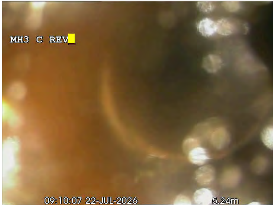
Photo: 78_4a, 00:00:00 5.3m, Joint displaced. Medium
