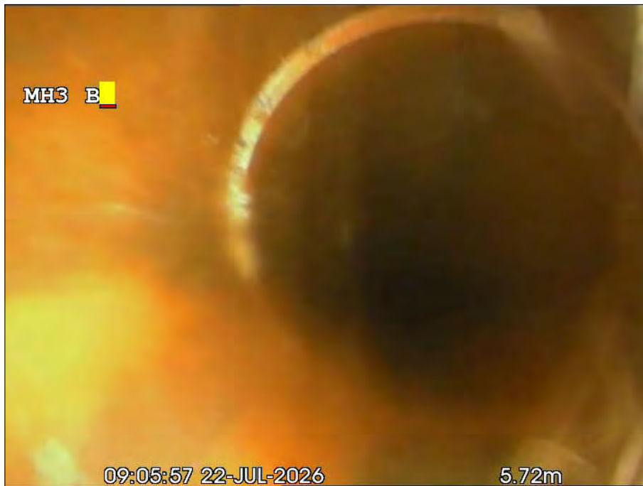
Photo: 7_9a, 00:00:00 5.8m, Joint displaced. Medium
