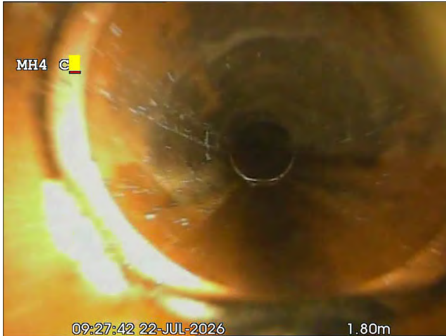
Photo: 17_4a, 00:00:00 1.9m, Joint displaced. Medium
