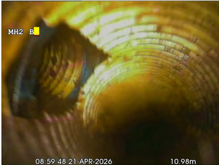
Photo: 283_8a, 00:00:00 11m, Connection, at 09 o'clock, dia 80 mm
