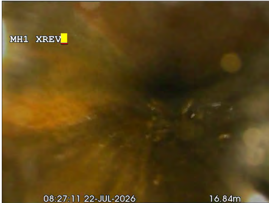
Photo: 21_8a, 00:00:00 17m, Debris silt, 10 % cross-sectional area loss, Start
