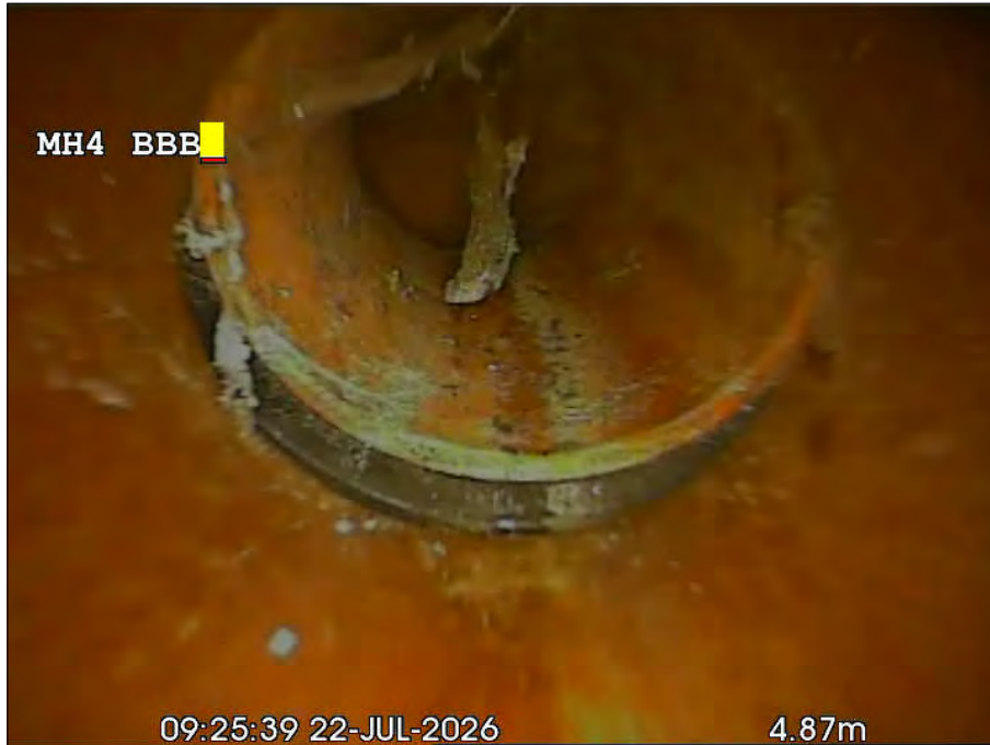
Photo: 112_6a, 00:00:00 5m, Joint displaced. Large
