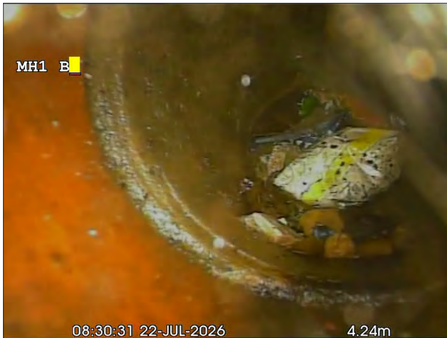
Photo: 234_9a, 00:00:00 4.3m, Joint displaced. Medium
