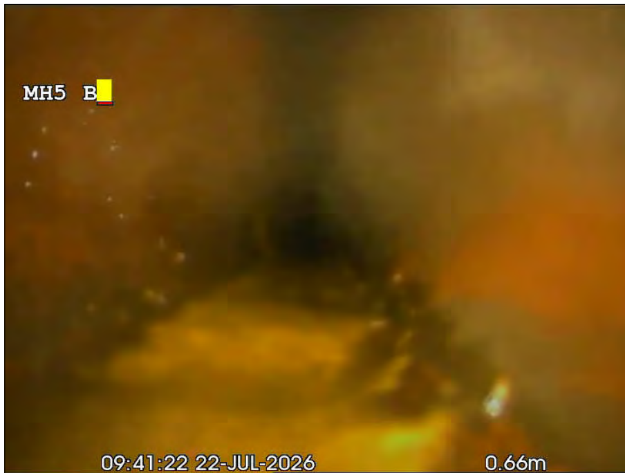
Photo: 23_5a, 00:00:00 0.15m, Debris silt, 10 % cross-sectional area loss, Start
