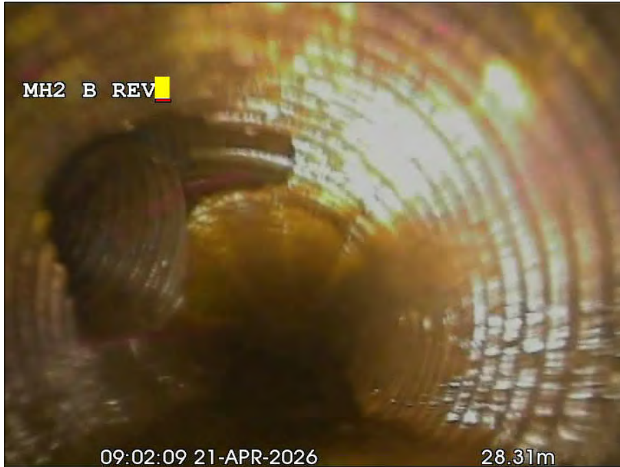
Photo: 32_12a, 00:00:00 28.5m, Connection, at 09 o'clock, dia 80 mm
