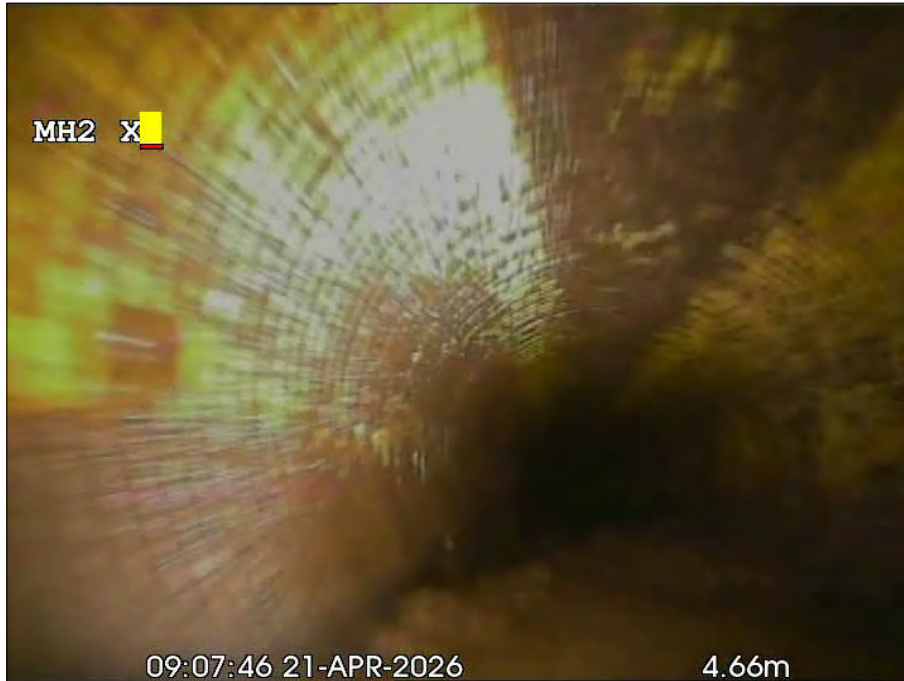
Photo: 301_4a, 00:00:00 4.6m, Debris silt, 5 % cross-sectional area loss
