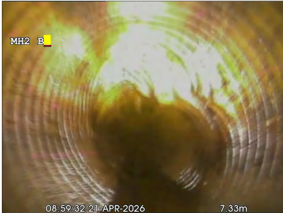
Photo: 281_6a, 00:00:00 7.5m, Sewer Deformed, 20 %
