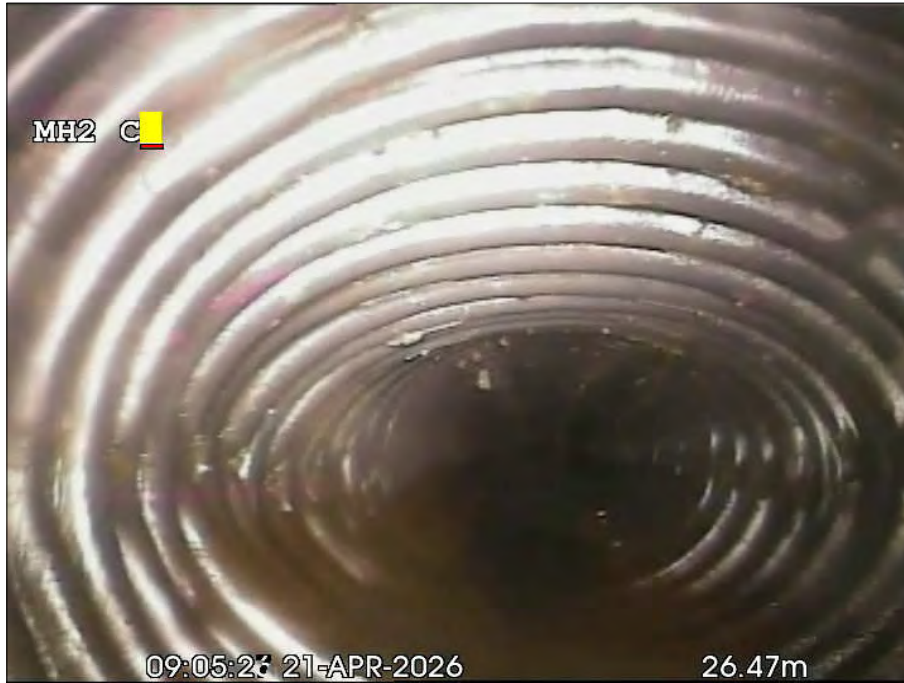
Photo: 296_6a, 00:00:00 26.5m, Sewer Deformed, 30 %
