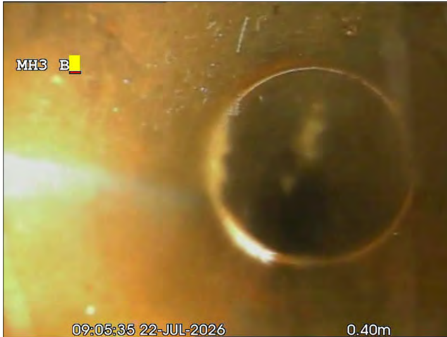
Photo: 7_4a, 00:00:00 0.5m, Joint displaced. Medium
