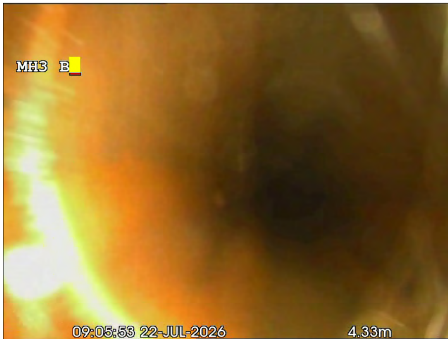
Photo: 7_7a, 00:00:00 4.4m, Joint displaced. Medium
