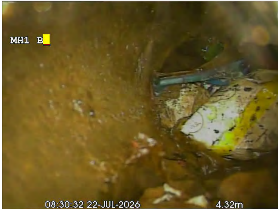
Photo: 235_10a, 00:00:00 4.4m, Obstruction, 60 % height/diameter loss
