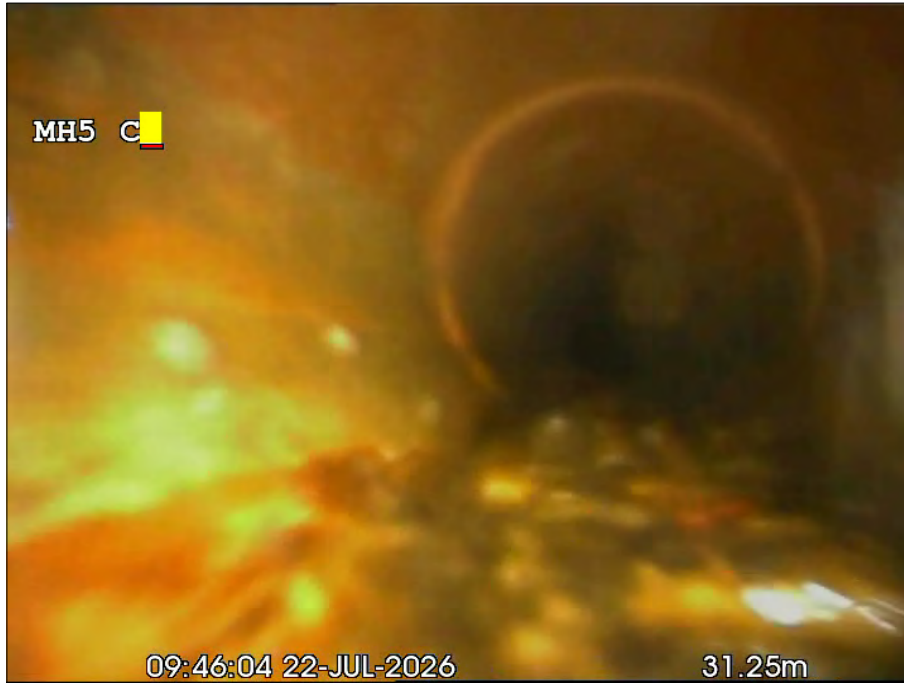
Photo: 24_12a, 00:00:00 31.3m, Debris silt, 5 % cross-sectional area loss, Start
