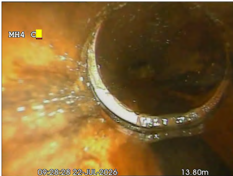
Photo: 17_7a, 00:00:00 14m, Joint displaced. Large
