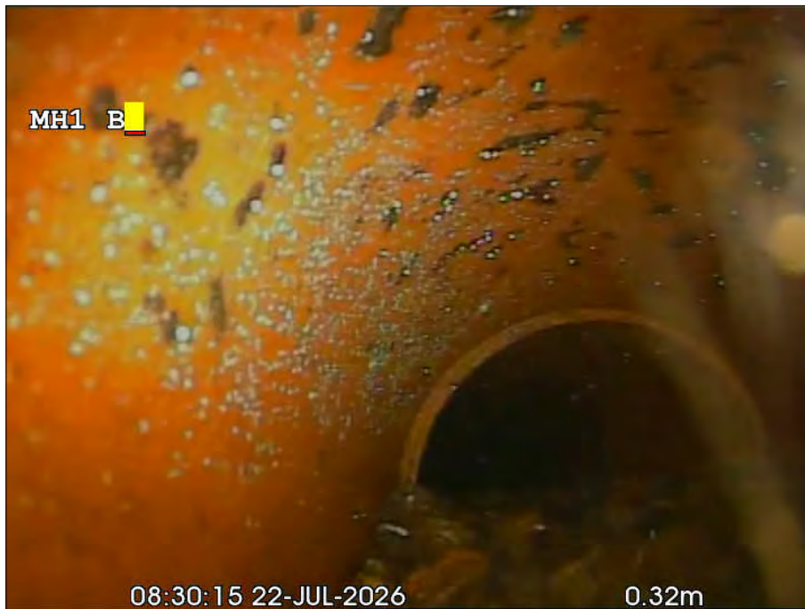
Photo: 231_5a, 00:00:00 0.7m, Debris, 40 % cross-sectional area loss, Changed
