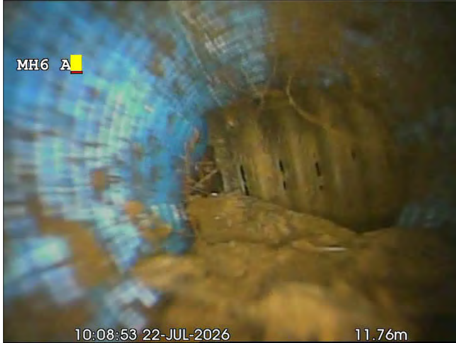
Photo: 28_12a, 00:00:00 12.55m, Obstruction, 95 % height/diameter loss
