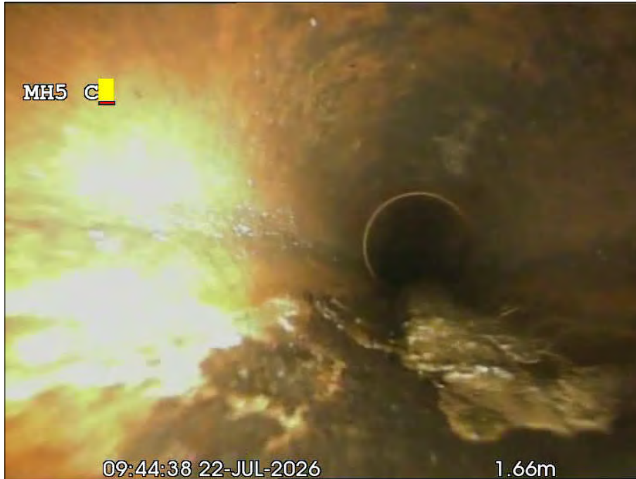
Photo: 169_3a, 00:00:00 0m, Debris silt, 10 % cross-sectional area loss, Start
