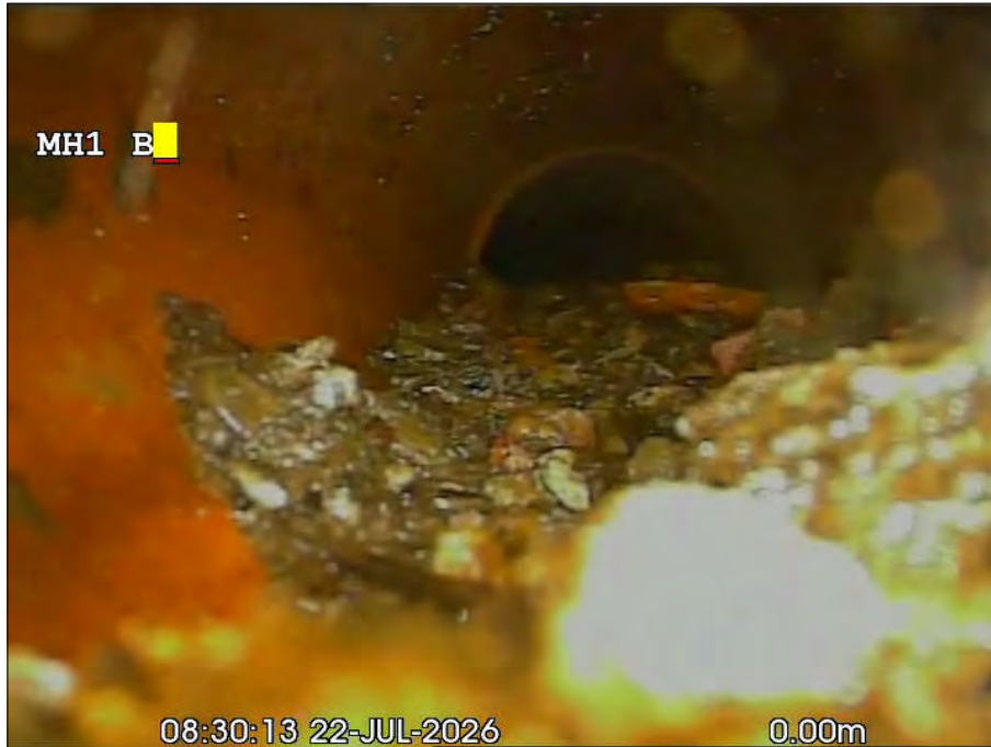
Photo: 230_4a, 00:00:00 0.1m, Debris, 10 % cross-sectional area loss, Start
