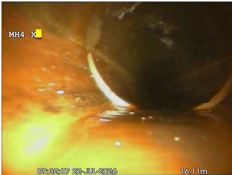
Photo: 147_8a, 00:00:00 16.4m, Joint displaced. Medium
