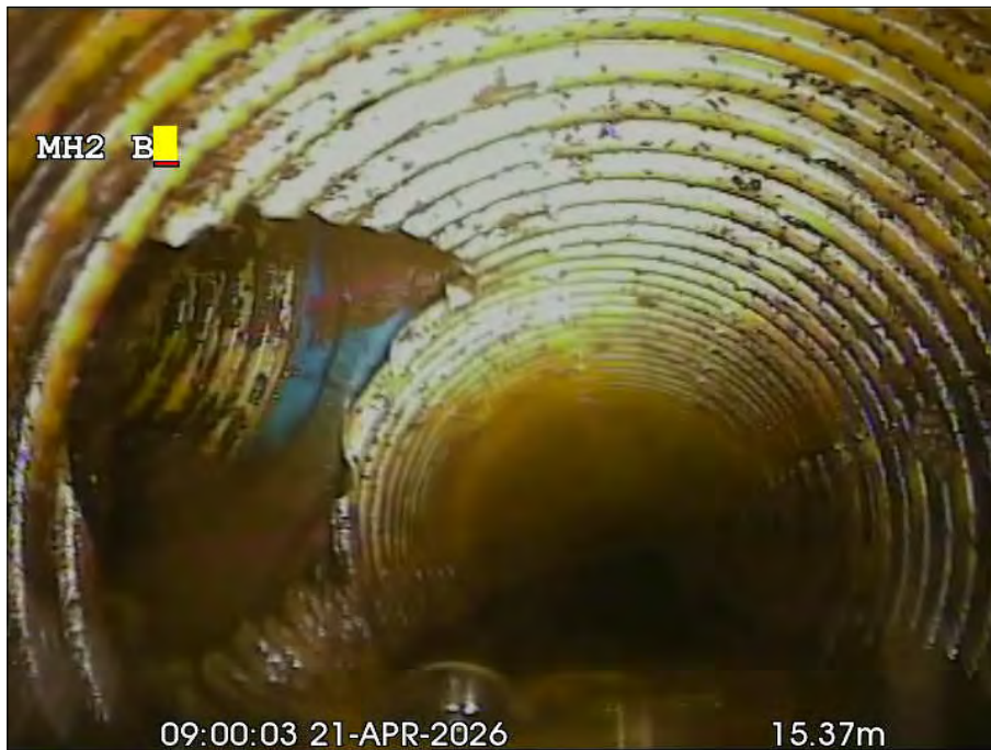
Photo: 284_9a, 00:00:00 15.4m, Connection, at 09 o'clock, dia 80 mm
