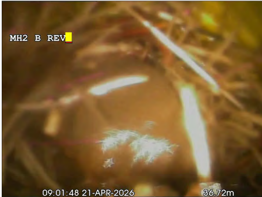
Photo: 32_14a, 00:00:00 36.7m, Mass Roots 95 % cross-sectional area loss
