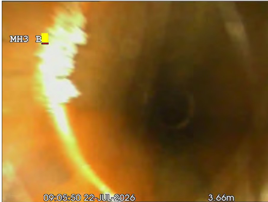
Photo: 7_6a, 00:00:00 3.7m, Joint displaced. Medium
