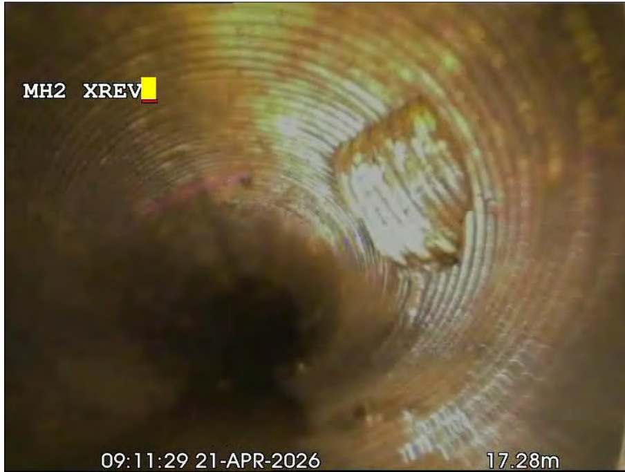
Photo: 314_11a, 00:00:00 17.4m, Connection, at 03 o'clock, dia 80 mm
