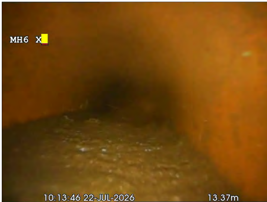
Photo: 30_7a, 00:00:00 13m, Debris silt, 25 % cross-sectional area loss, Changed
