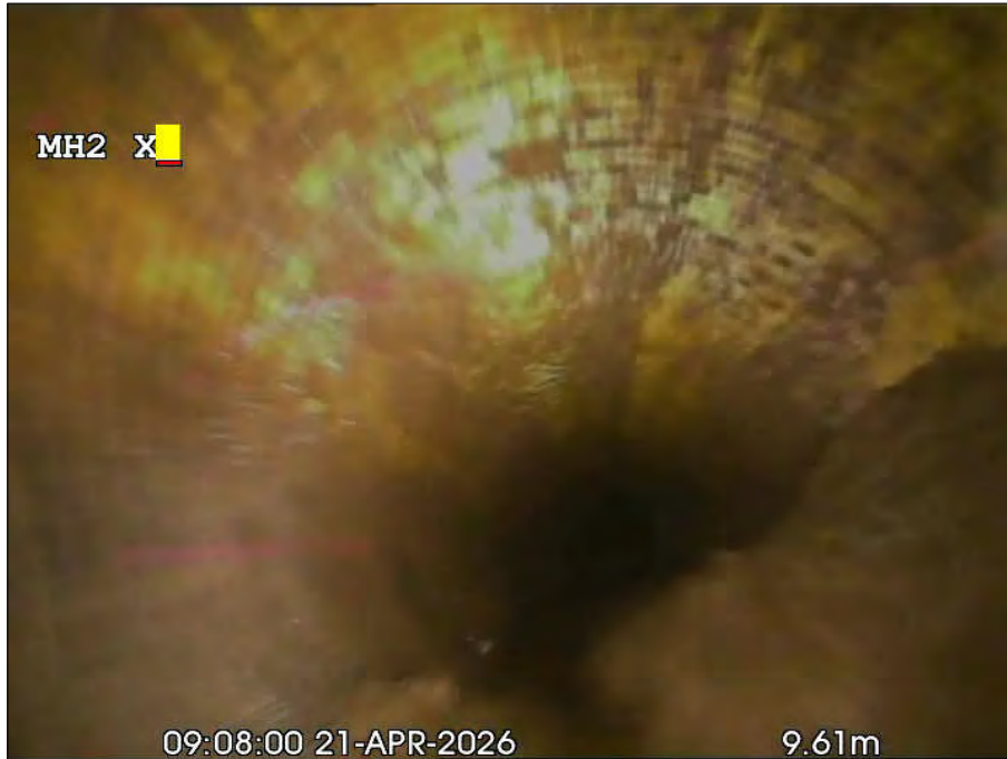
Photo: 305_8a, 00:00:00 9.6m, Debris silt, 20 % cross-sectional area loss, Start
