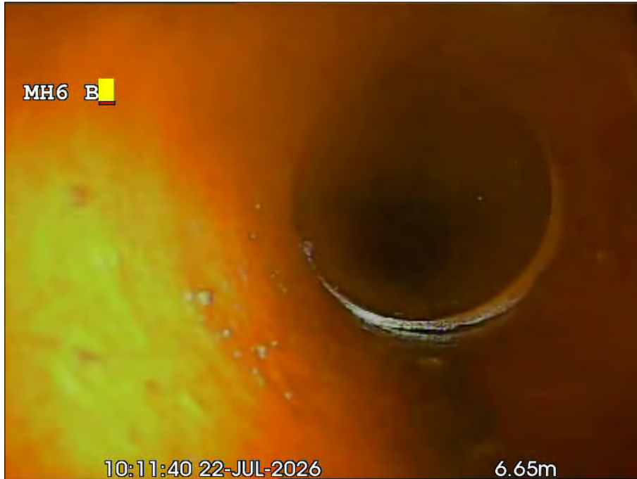
Photo: 29_6a, 00:00:00 6.8m, Joint displaced. Medium
