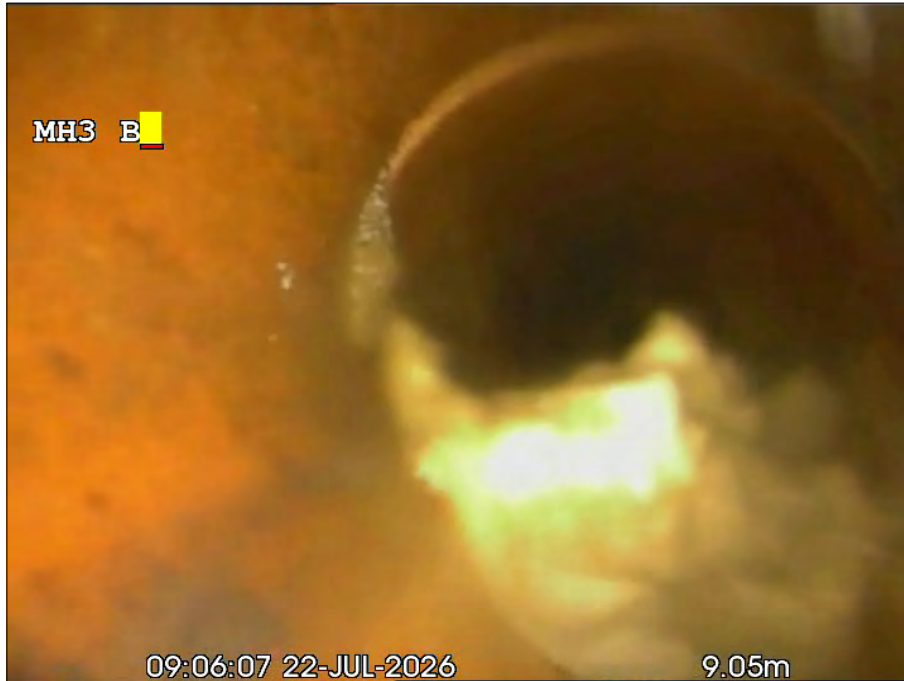
Photo: 62_12a, 00:00:00 9.1m, Debris silt, 25 % cross-sectional area loss
