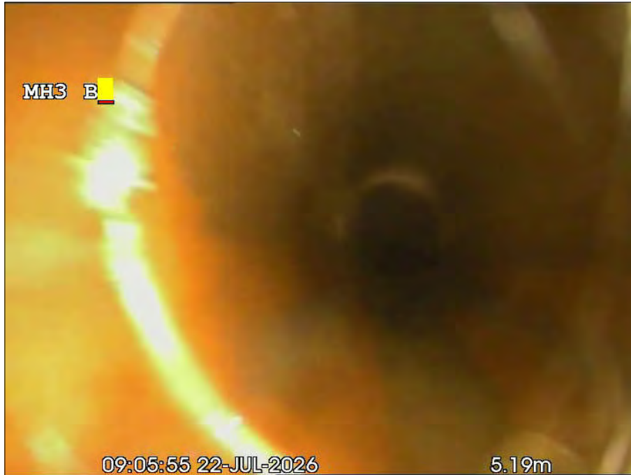
Photo: 7_8a, 00:00:00 5.1m, Joint displaced. Medium
