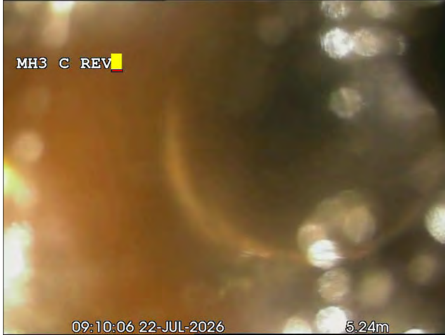
Photo: 10_7a, 00:00:00 7.6m, Line of Sewer deviates down
