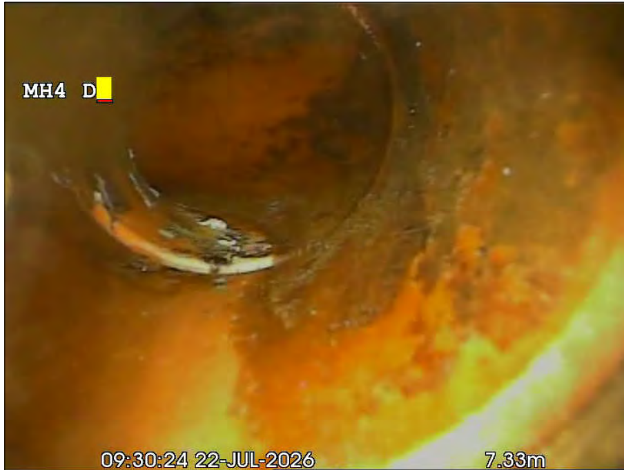
Photo: 18_8a, 00:00:00 7.6m, Joint displaced. Medium
