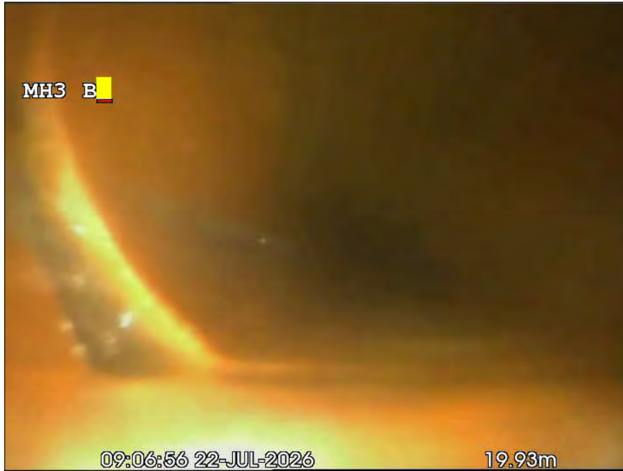
Photo: 7_16a, 00:00:00 20m, Joint displaced. Large
