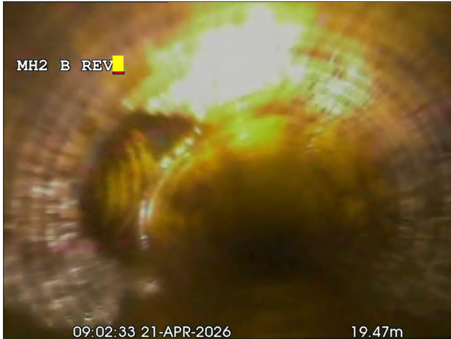
Photo: 290_10a, 00:00:00 19.5m, Connection, at 09 o'clock, dia 100 mm
