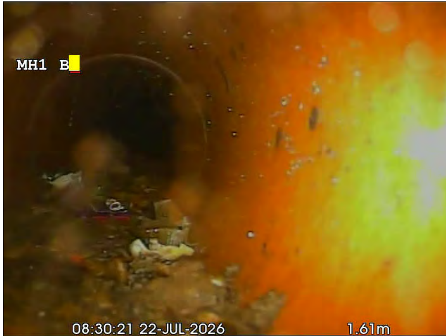
Photo: 232_6a, 00:00:00 1.6m, Debris, 10 % cross-sectional area loss, Changed
