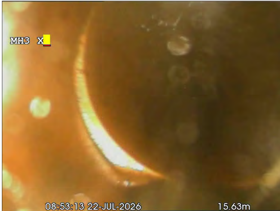
Photo: 11_6a, 00:00:00 15.7m, Joint displaced. Medium
