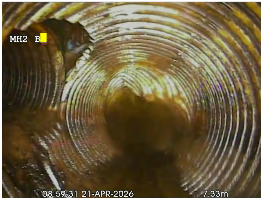
Photo: 280_5a, 00:00:00 7.3m, Connection, at 09 o'clock, dia 80 mm
