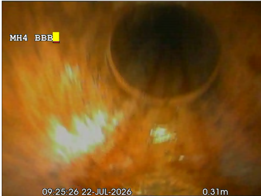
Photo: 110_4a, 00:00:00 0.4m, Line of Sewer deviates up
