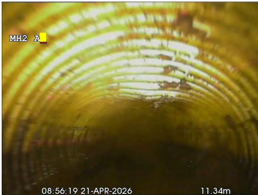
Photo: 270_5a, 00:00:00 11.4m, Sewer Deformed, 5 %
